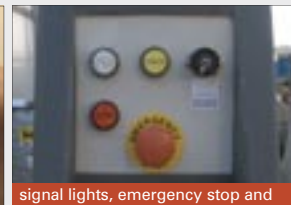
signal lights, emergency stop and connection plug for handcontrol on all columns
